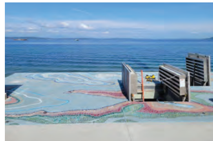
SPU converted the airlift-type pipe station to a more standard pump station, which will reduce the risk of failure, improve system reliability and performance and reduce maintenance costs. (Photo credit: Seattle Public Utilities)
