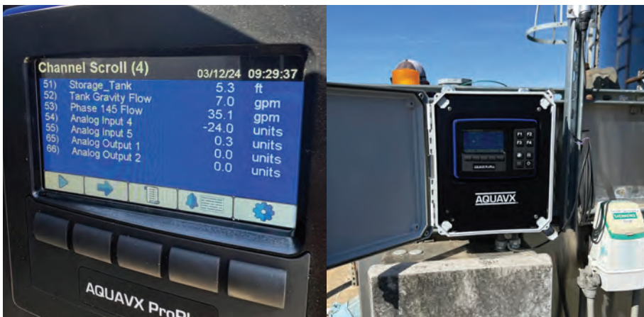
The continuous statistics have also enabled the town to perform predictive analytics and schedule maintenance activities proactively.
