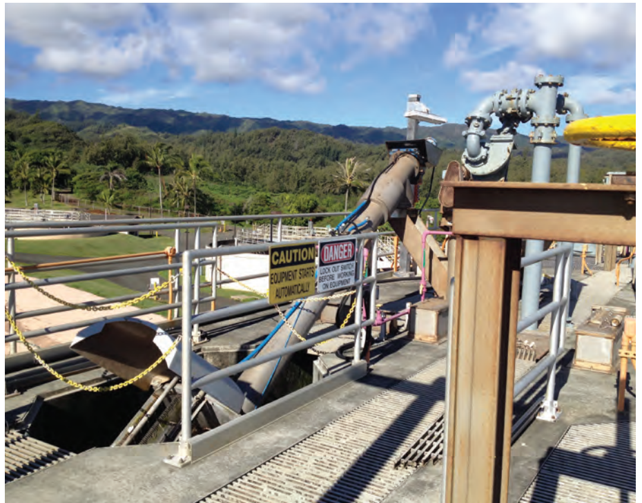
Lakeside's latest installation in Hawaii includes a Raptor FalconRake Bar Screen and an In-Line Grit Collector.
