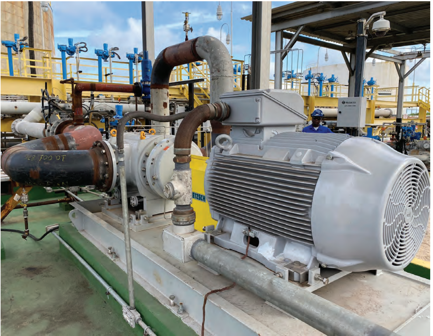
As the 4NS can handle highly viscous media, no diesel injection was required, which in turn resulted in a significant cost reduction.
