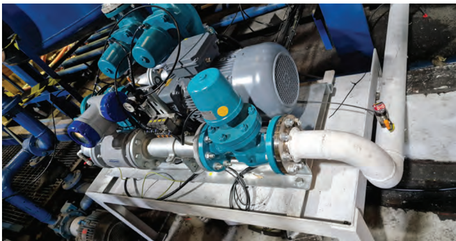
The new Borger pump at Moove, which is for a three-bar application.
