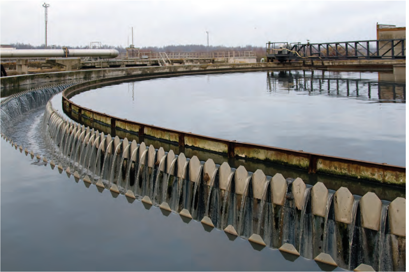
The twofold nature of wastewater-treatment facilities—treating fouled wastewater and providing clean water—require pumps that can handle a variety of fluids.
