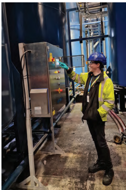
At Moove, Borger carried out a full site test, running different configurations to determine the best operating modes.
