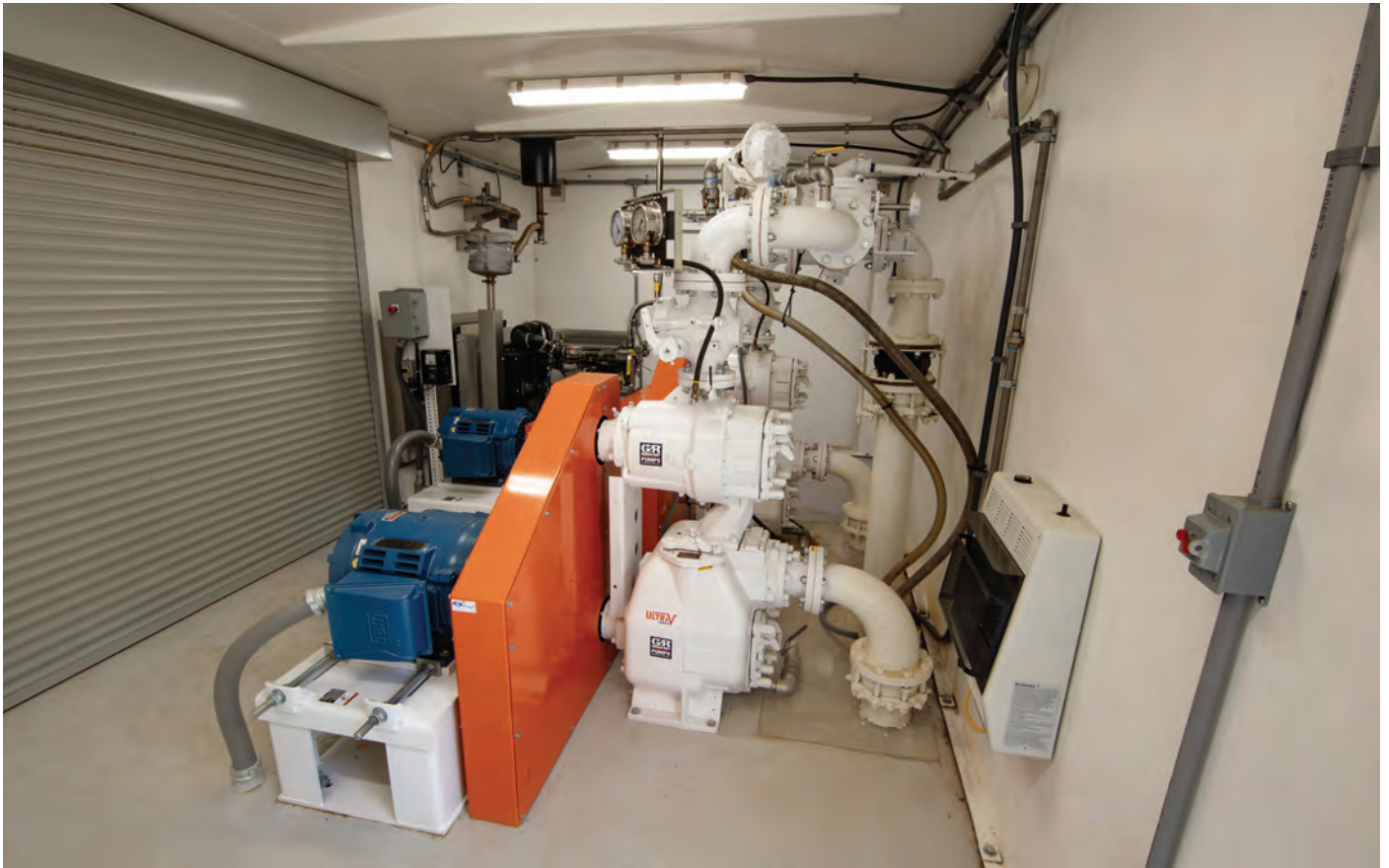
The enlarged size of modular enclosures provides added space for performing routine pump maintenance while shielding operators from external conditions. Oversized roll-up doors allow access to station components should heavier-duty lifting equipment be required.
